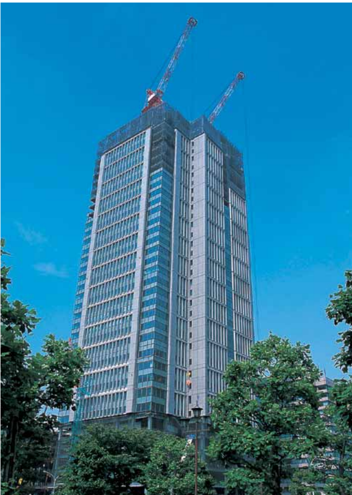
The Marunouchi Building under construction, which is scheduled for completion in August 2002.
